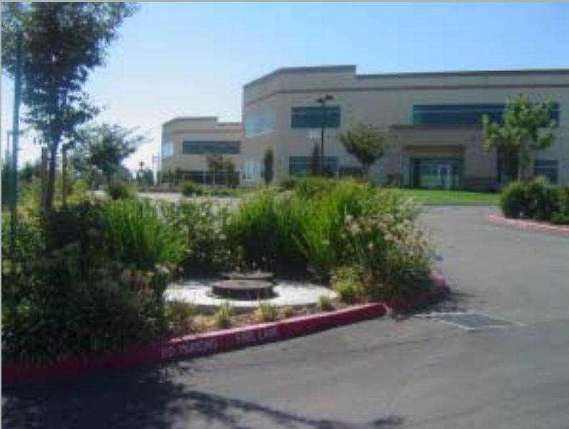
Swirl Separator in Parking Lot
