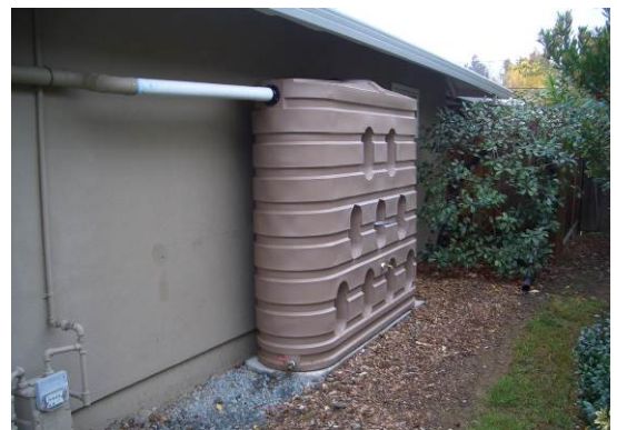
Large unit installed at a single family residence.
