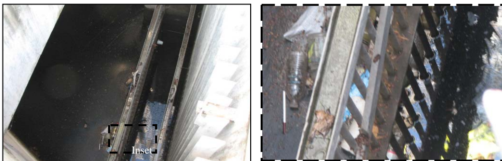
Photo 3 - Matadero Pump Station - (a) Small and Large Trash Racks; (b) Close-up of Small Trash Rack
