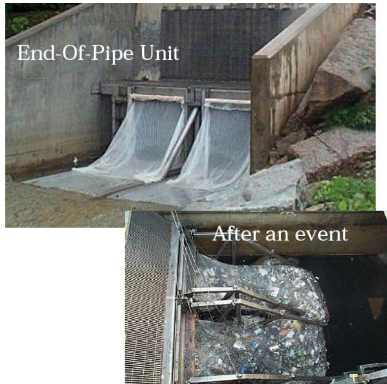
Photo 14 – Sample End-of-Pipe Trash Nets (a) Empty and (b) Full of Trash
