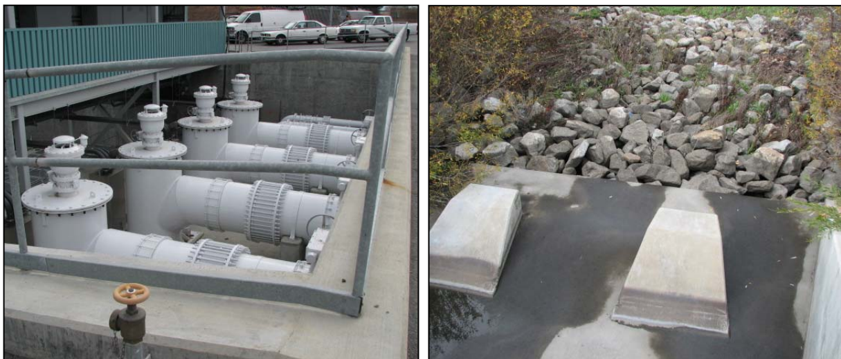
Photo 6 – Rincon 2 Pump Station (a) View of Pumps; (b) Discharge Structure
