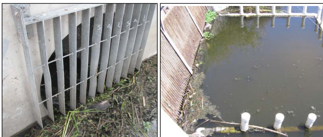
Photo 1 –Trash Racks - (a) Wrigley-Ford Creek culvert; (b) City of Sunnyvale Pump Station #1
