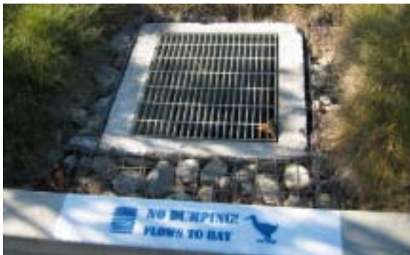
Storm drains are clearly labeled with an educational “no dumping” message.
